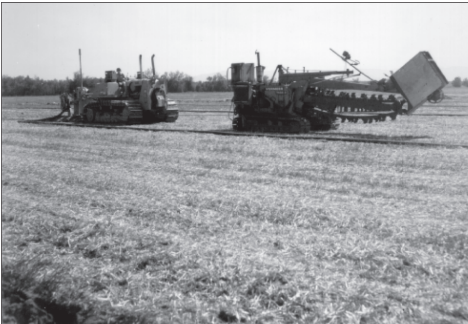
Figure 26.—Tile drainage. Specialized trenching machines install continuous PVC drain tiles into the soil. The gradient of the tile lines is carefully controlled with laser beams to ensure good water flow. The depth of the tile lines and the spacing between them depend on the properties of the soil and the depth to the water table.
